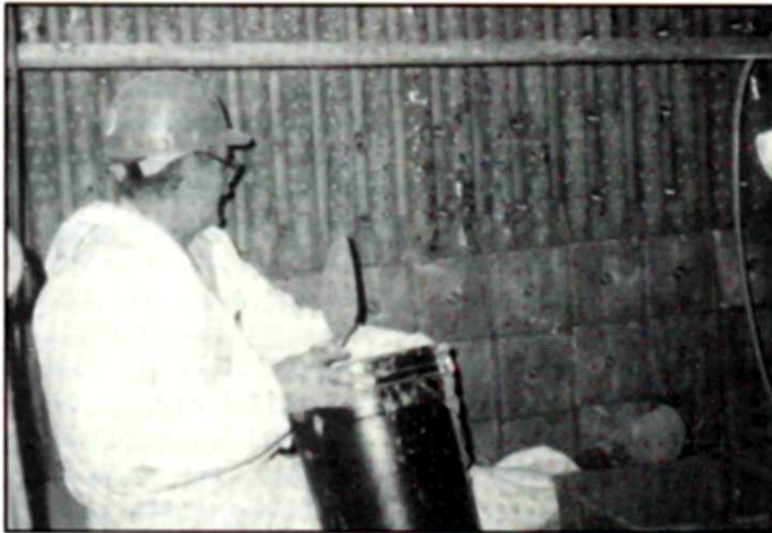
Metal bolts are welded directly to the metal membrane of the water-walls as a first step in installing the new tile refractory system. Mortar is then applied as the tiles are set in place.
